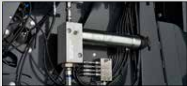
Automatic greasing system for roller bearings
